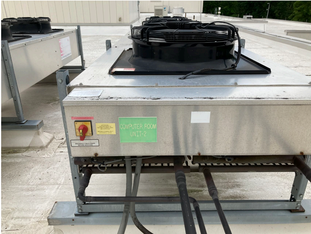
ROOF TOP COOLING UNIT
